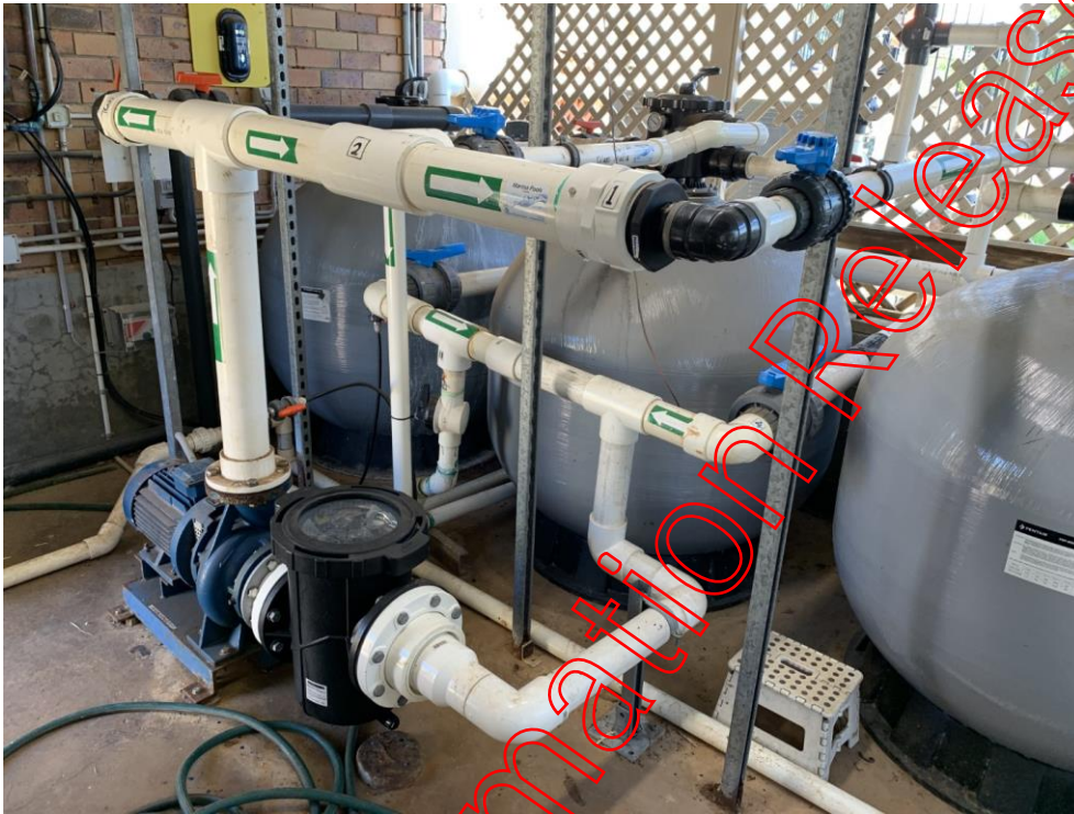
Figure 93: 25m Pool Pump and Filters
