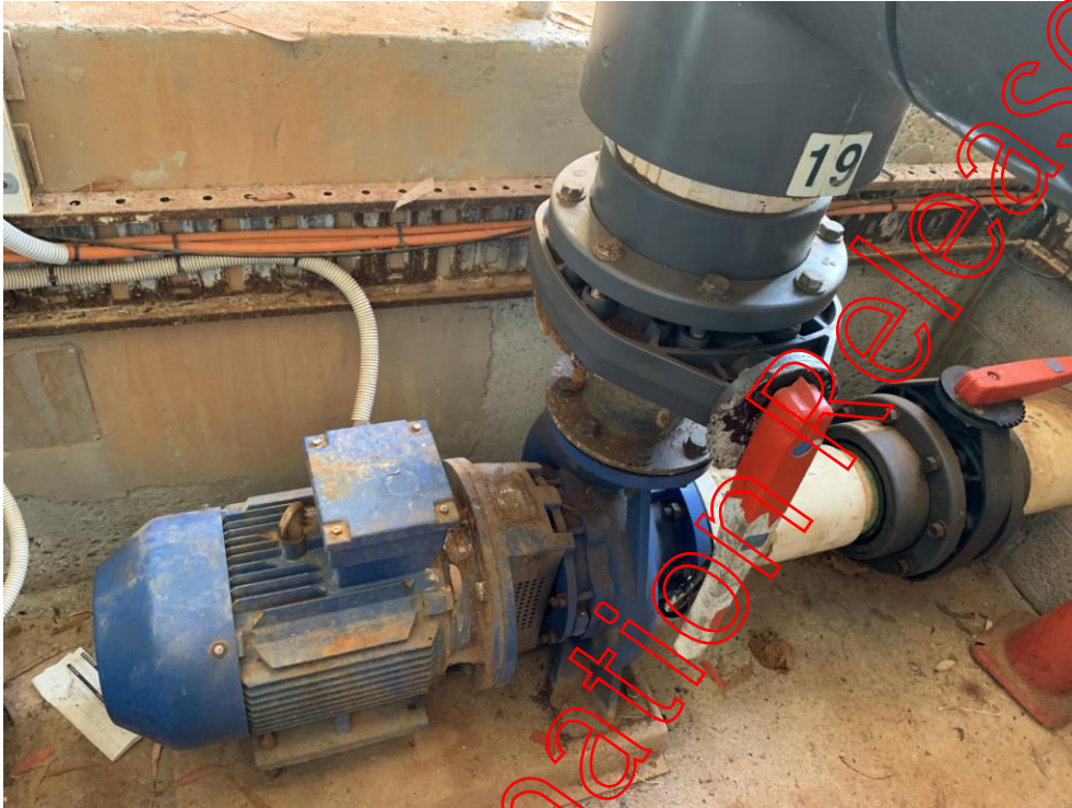
Figure 129: River pump 1, poor access
