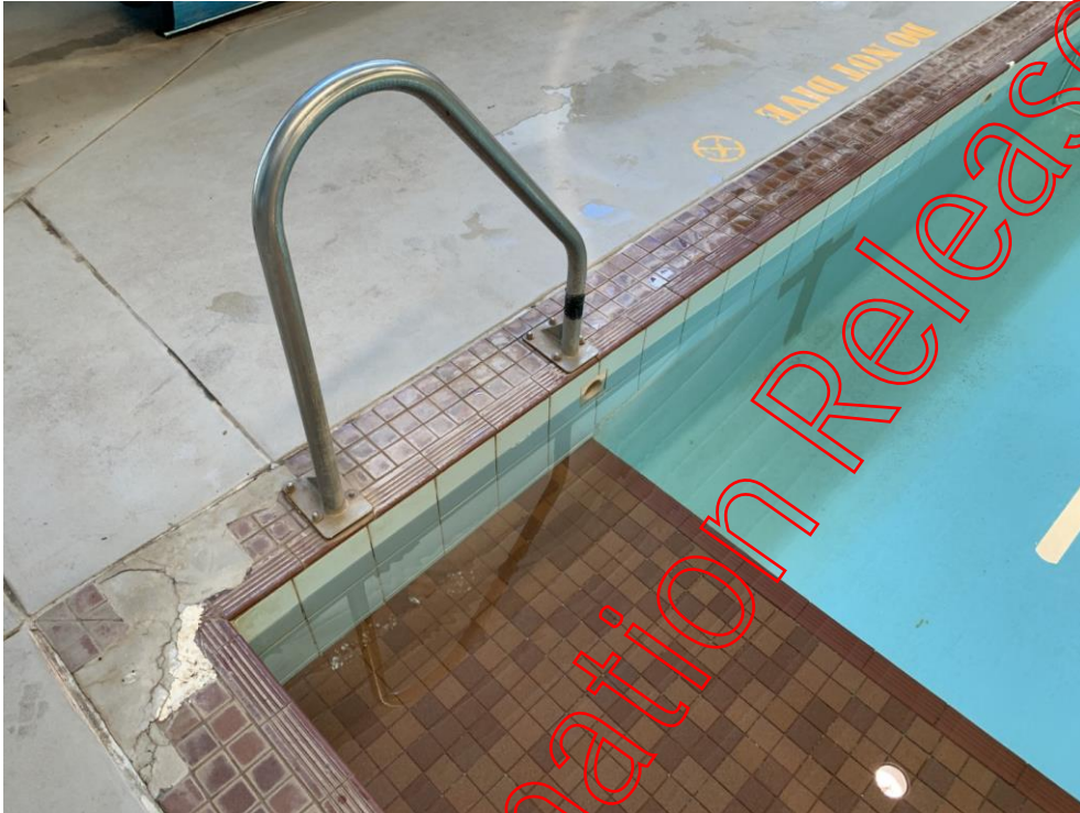
Figure 24: Damaged tiling, non-compliant access
