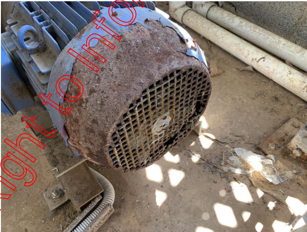
Figure 101: Poor condition pump motor
