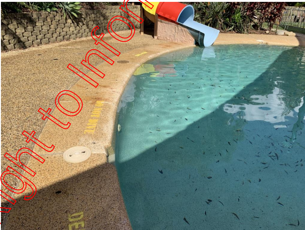
Figure 40: Cracks in coping
