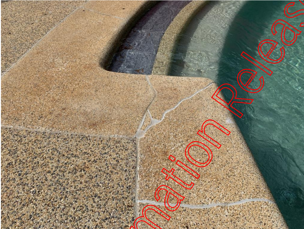
Figure 47: Numerous cracks in pool coping
