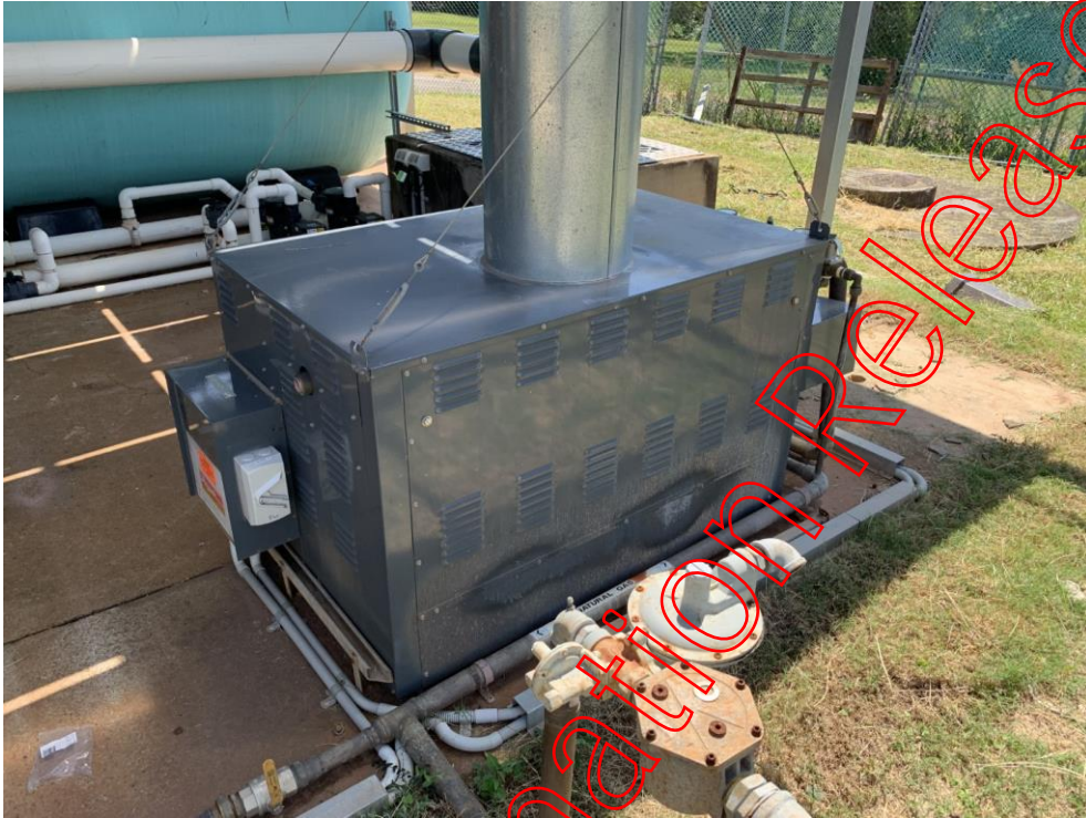
Figure 71: inefficient gas boilers
