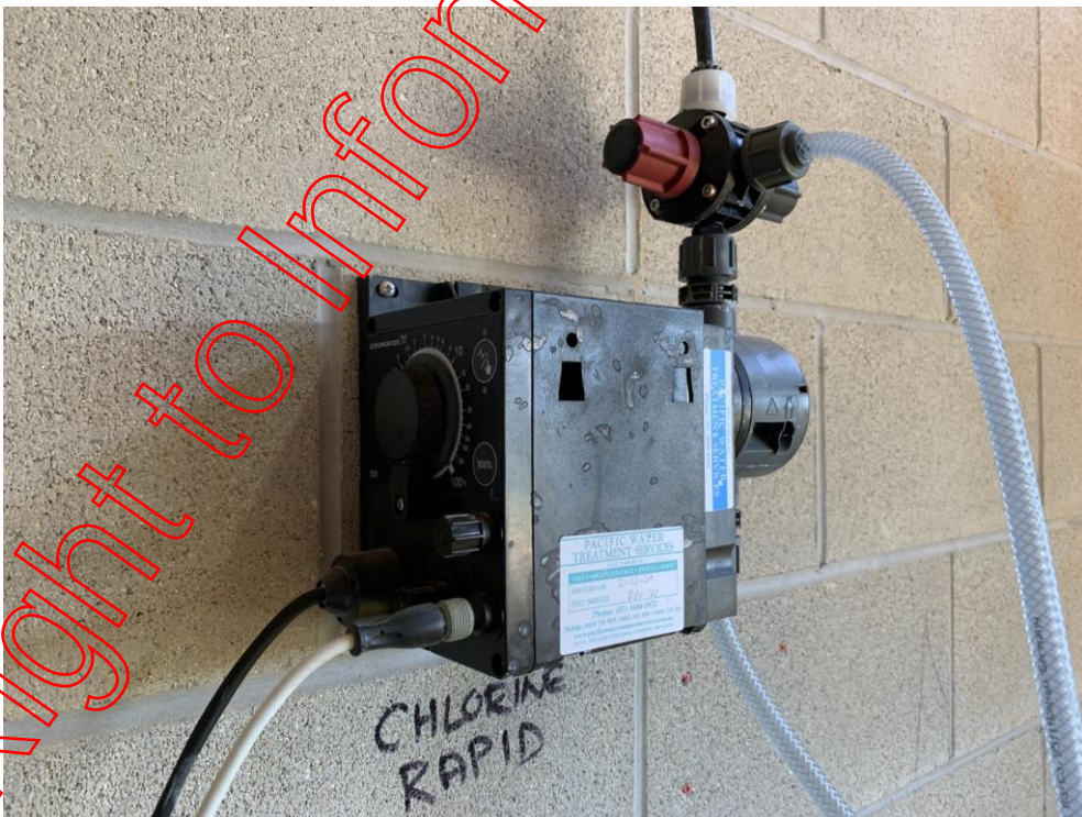
Figure 134: Chlorine pump installed at high level
