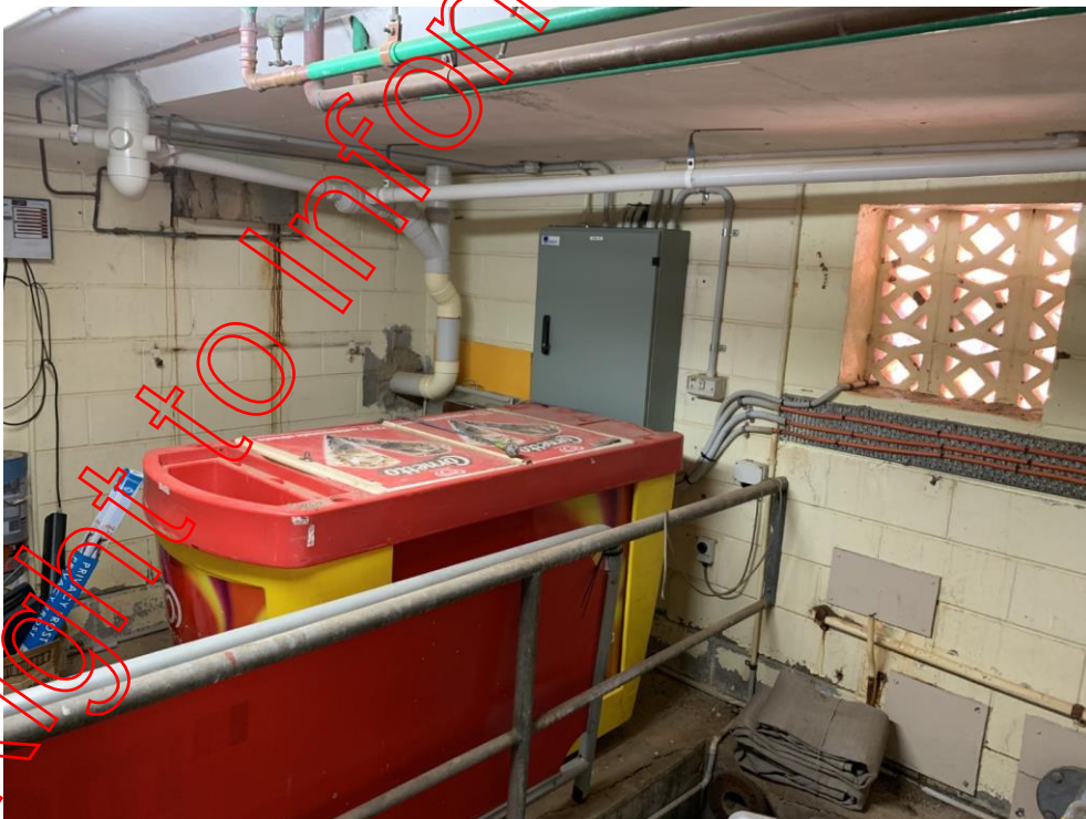
Figure 86: Obstructed main distribution board
