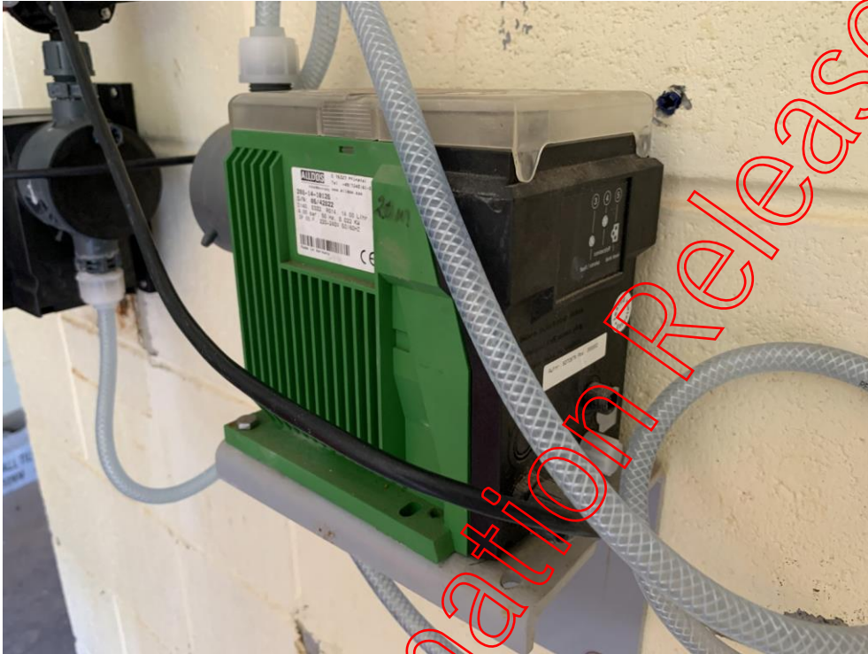
Figure 106: Chlorine dosing pump with no multifunction valve
