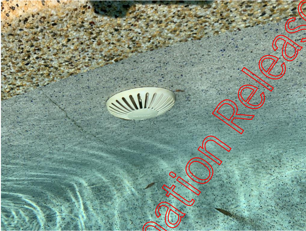
Figure 39: Older safety suction, crack in wall
