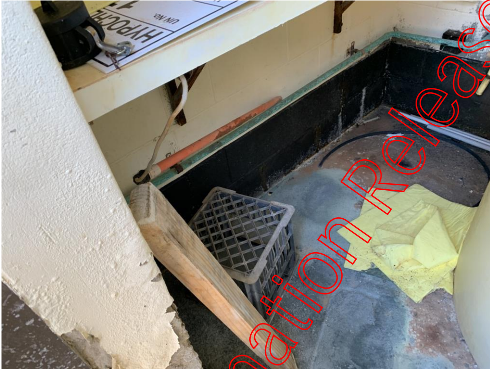
Figure 91: Poor condition bund with debris
