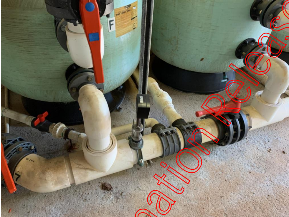
Figure 117: Flow meter installed in wrong location
