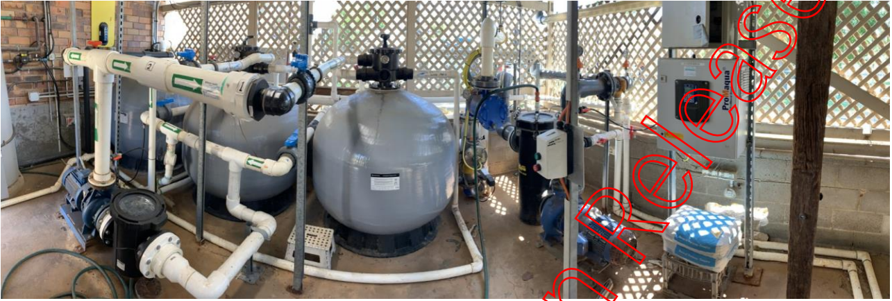
Figure 75: Poor access through equipment room
