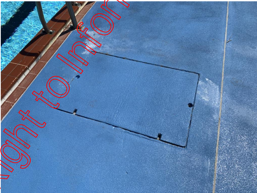
Figure 8: Heavy balance tank lid
