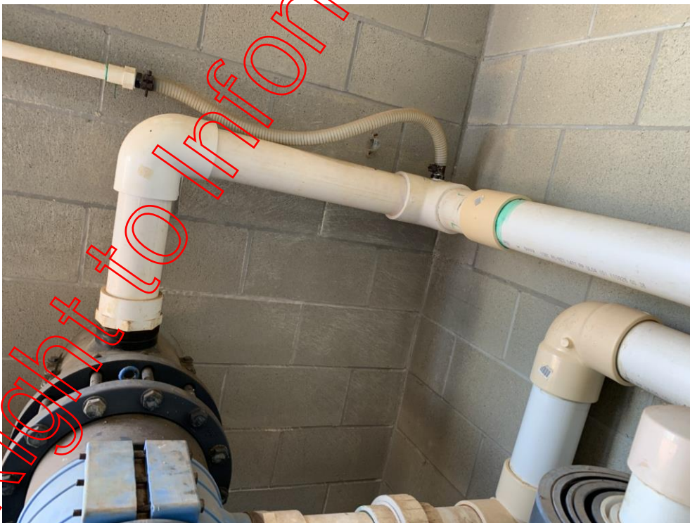
Figure 130: Filtration suction and return connections from river pump
