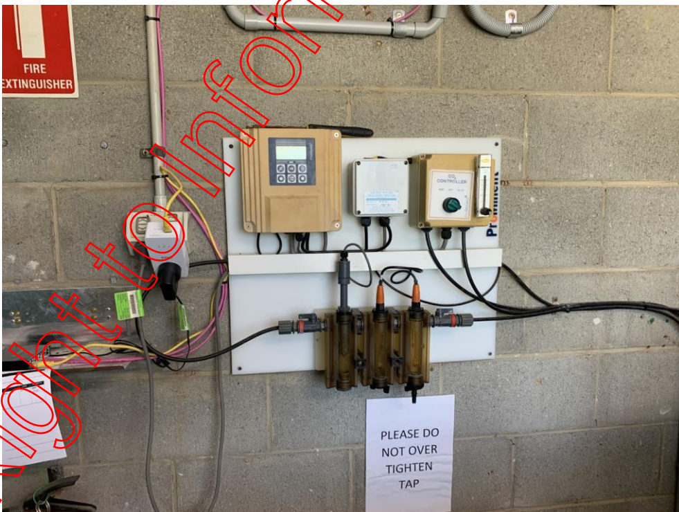
Figure 70: Obsolete chemical controller
