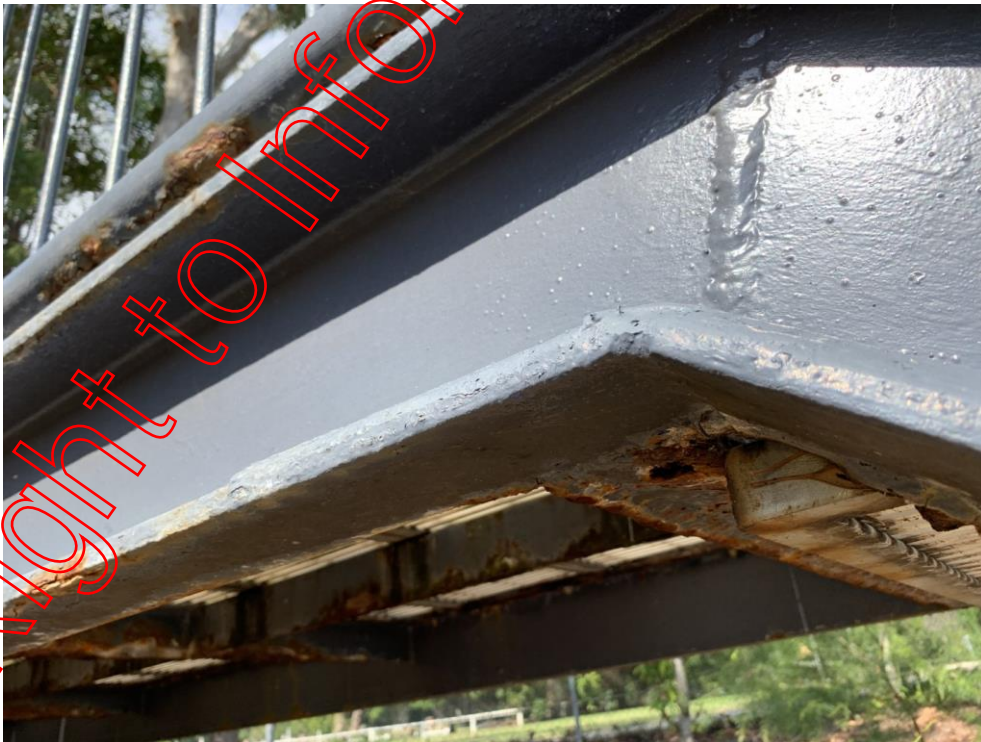
Figure 43: Rust under slide access way
