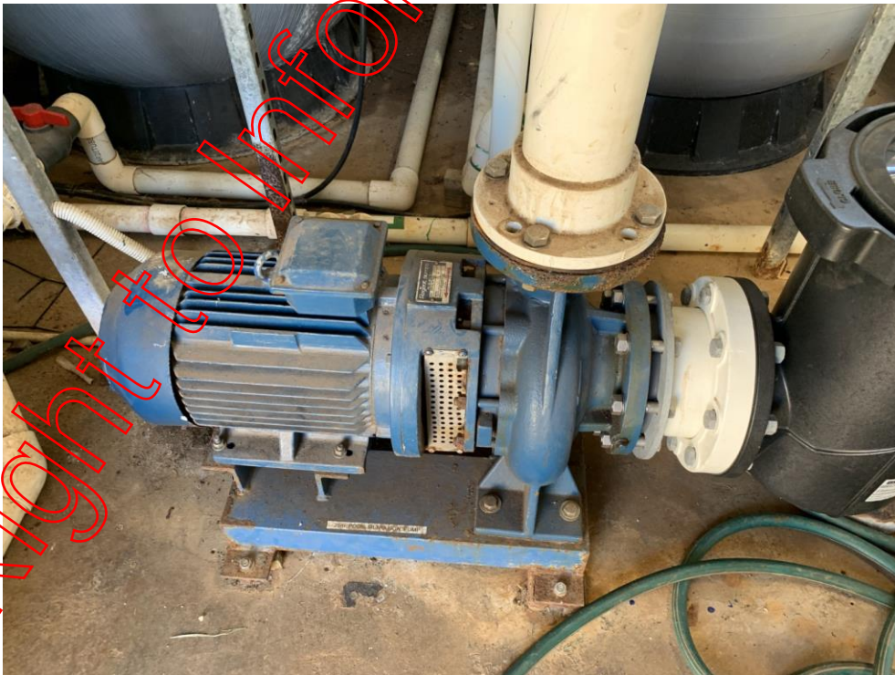
Figure 95: Filtration pump installed direct to slab, rusty baseplate
