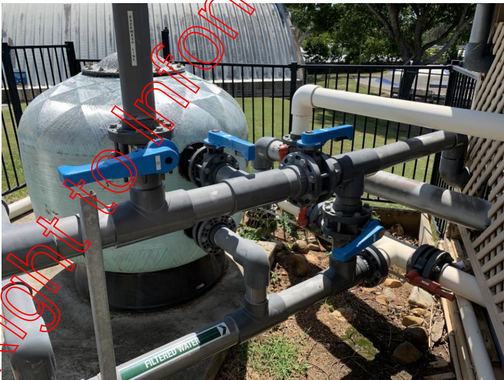
Figure 78: Poorly installed and supported pipe
