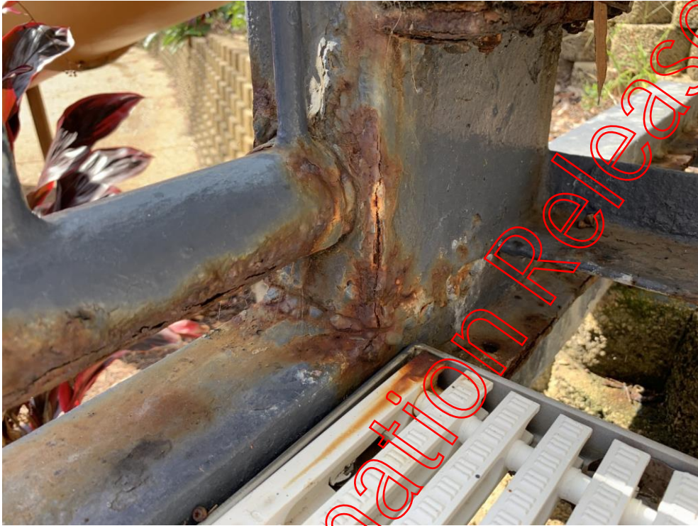
Figure 44: Rust in slide access way
