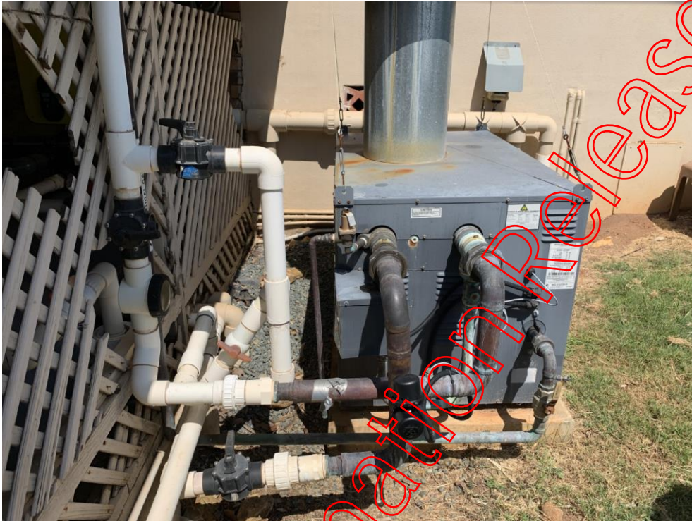
Figure 77: Poorly installed and supported pipe
