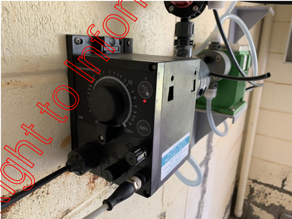
Figure 97: Chlorine dosing pump, overpressure line discharging to room
