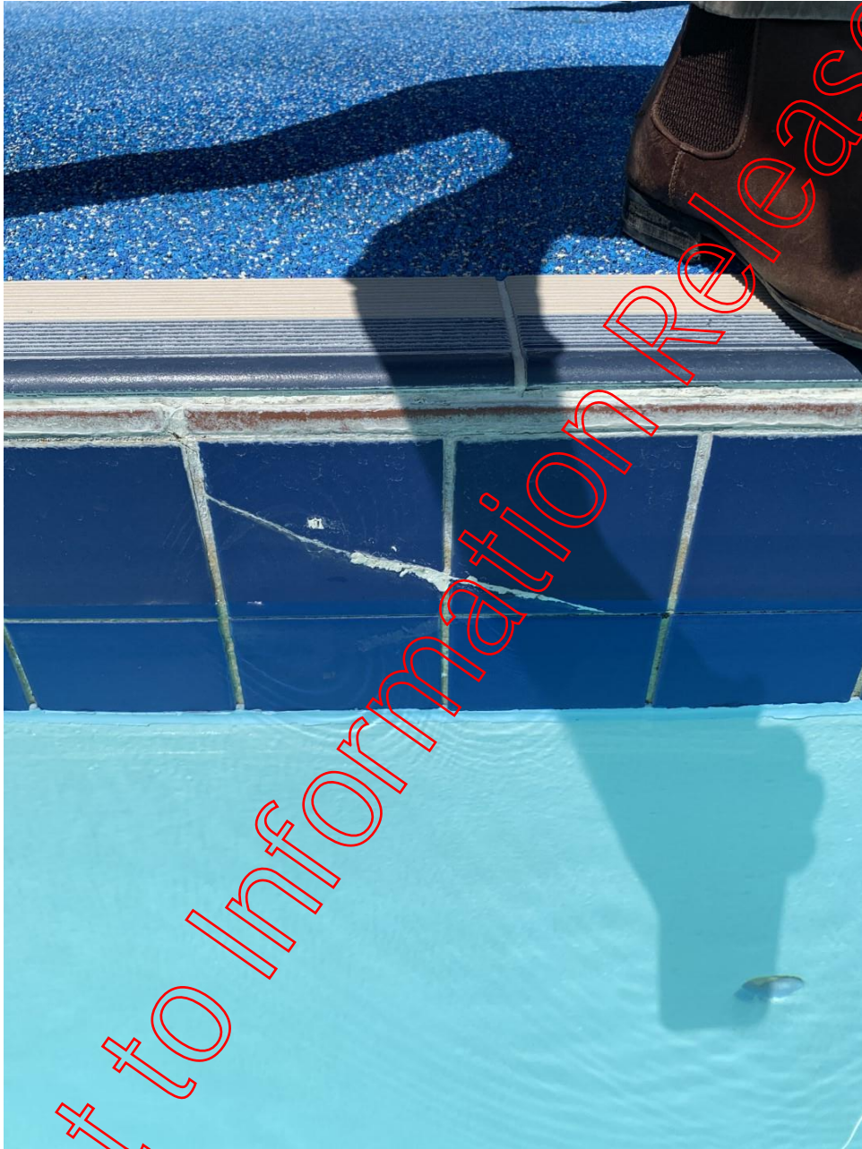
Figure 15: Crack in structure
