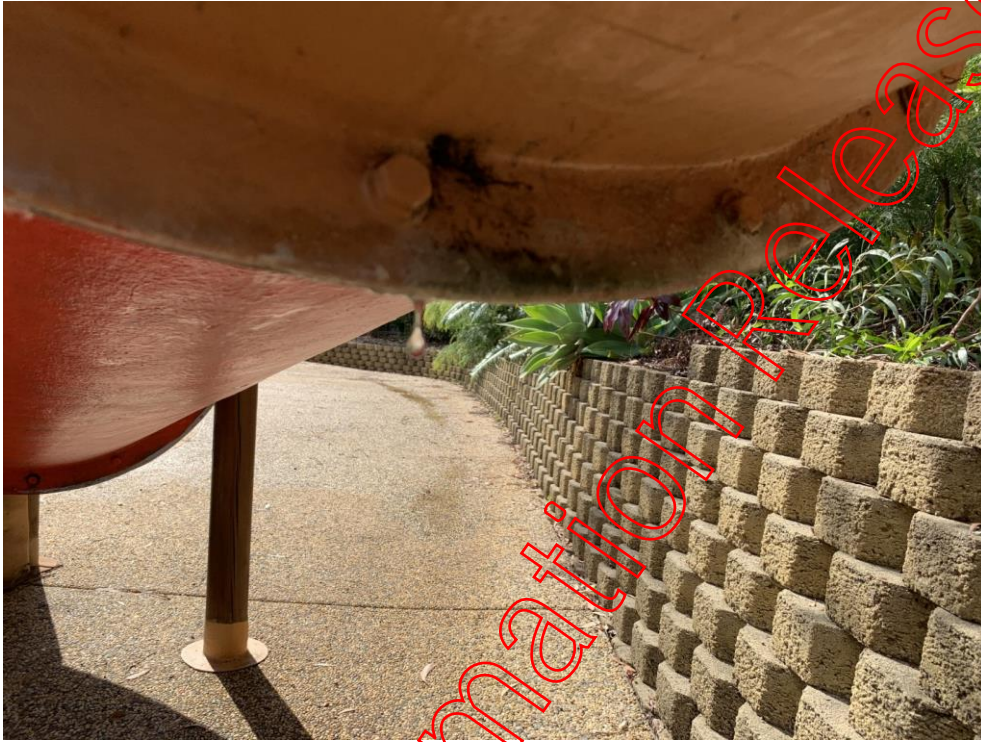
Figure 42: Leaks from slide flume
