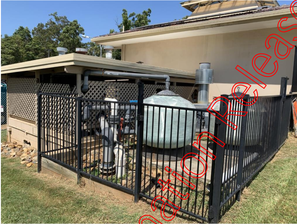
Figure 81: UV Degraded external equipment
