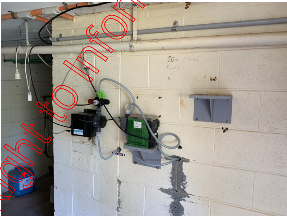
Figure 84: Unlabeled equipment in equipment room, loose extension cord
