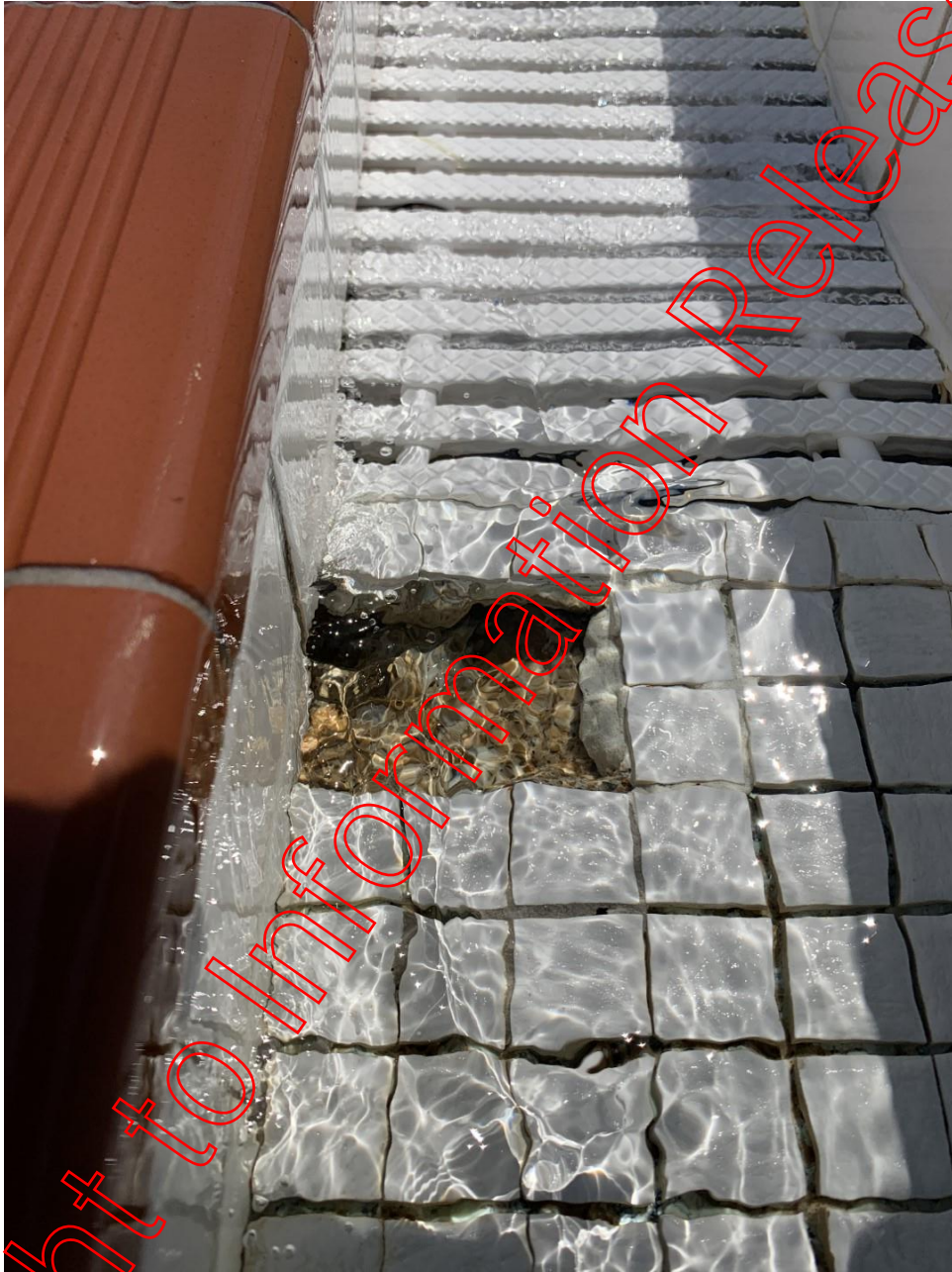
Figure 4: Failed tiling in gutter floor
