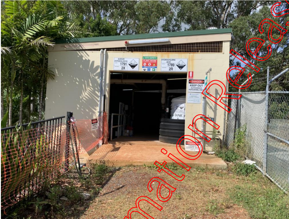
Figure 108 Western Equipment Room
