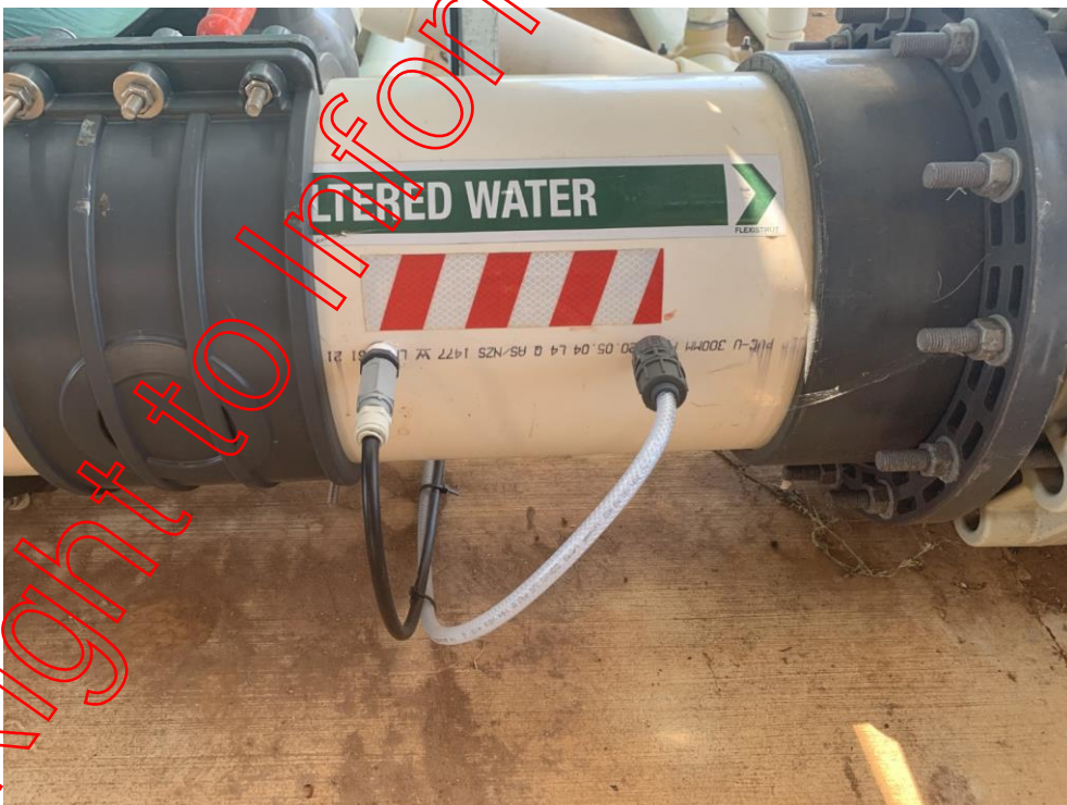
Figure 72: Unlabeled chemical injectors
