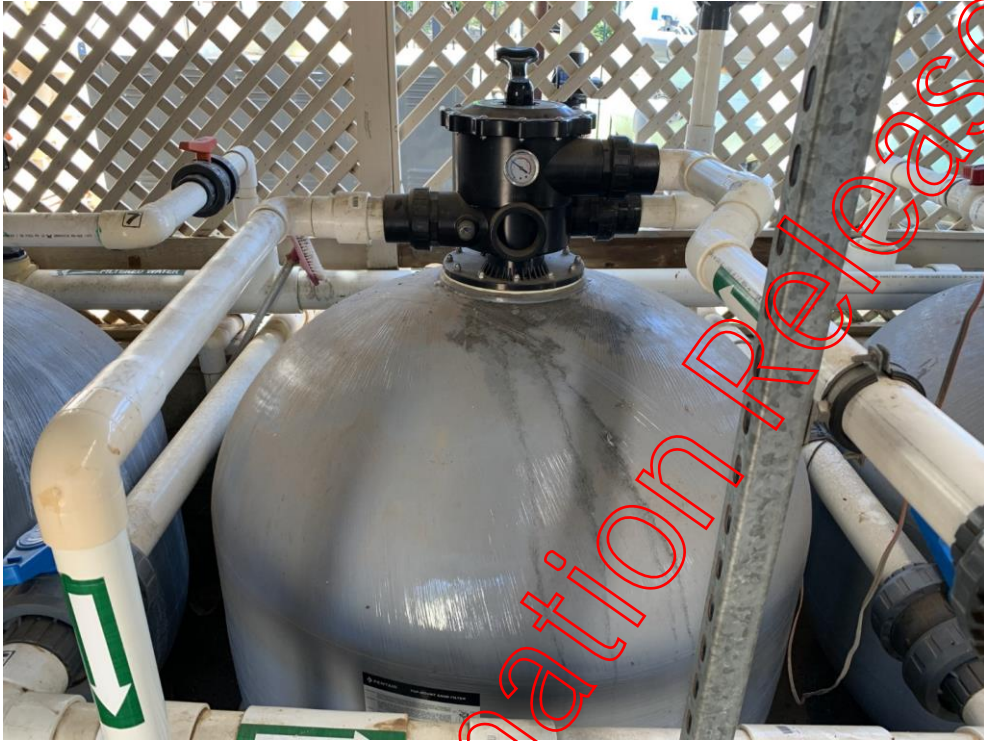
Figure 79: Poorly installed pipework, inaccessible multiport valve
