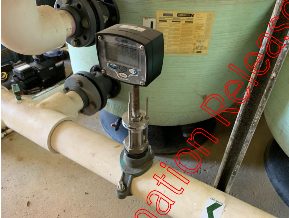
Figure 133: Flow meter installed upstream of filter
