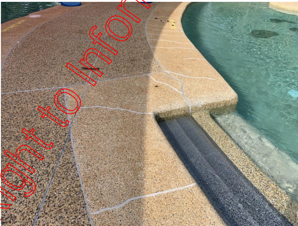
Figure 54: Sealed cracks at overflow chamber
