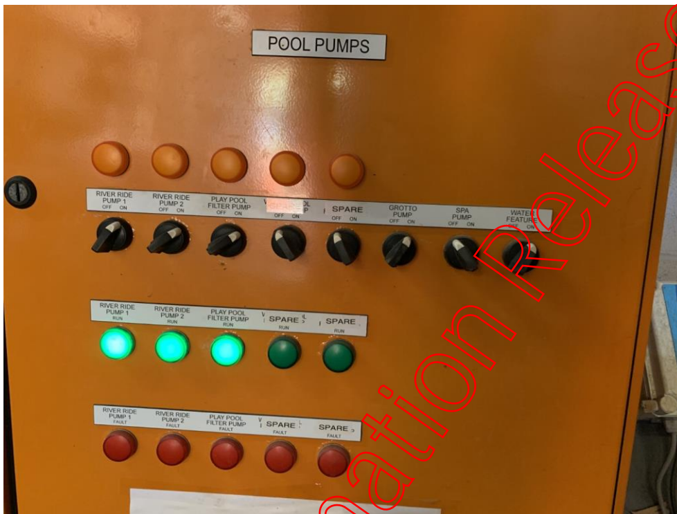
Figure 121: Obsolete switchgear for spa in board
