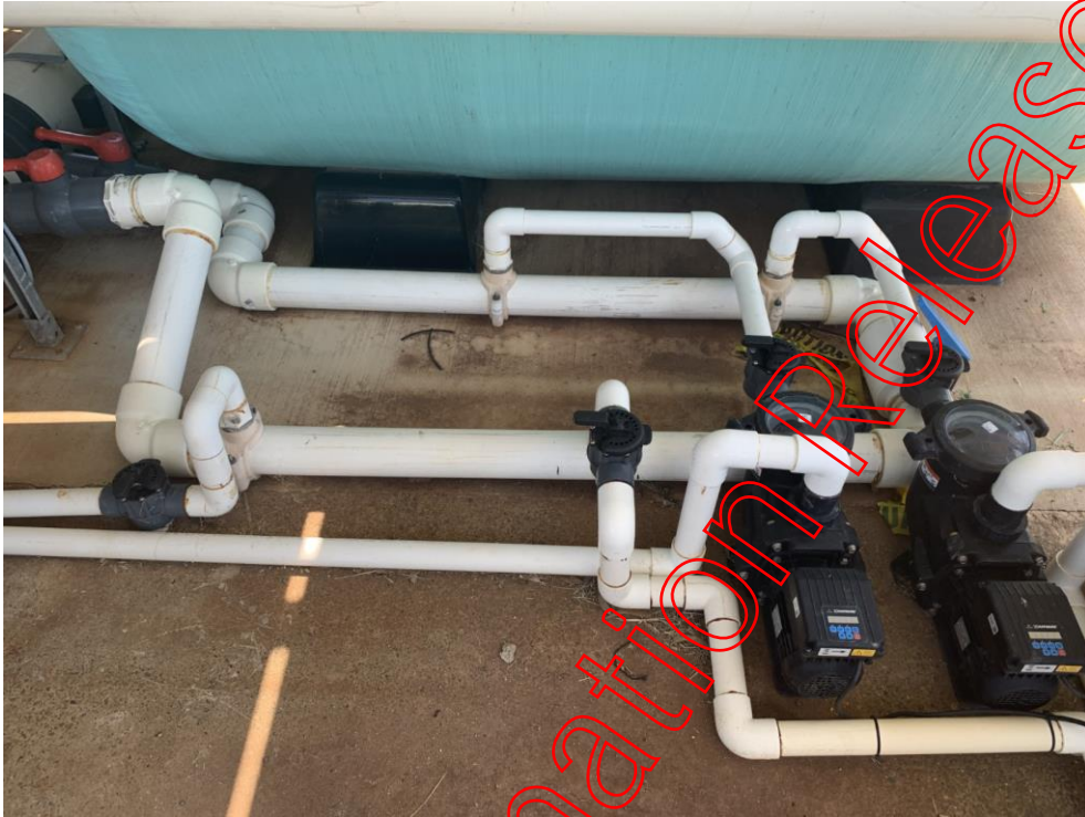
Figure 63: Unlabeled poorly configured heater pipework
