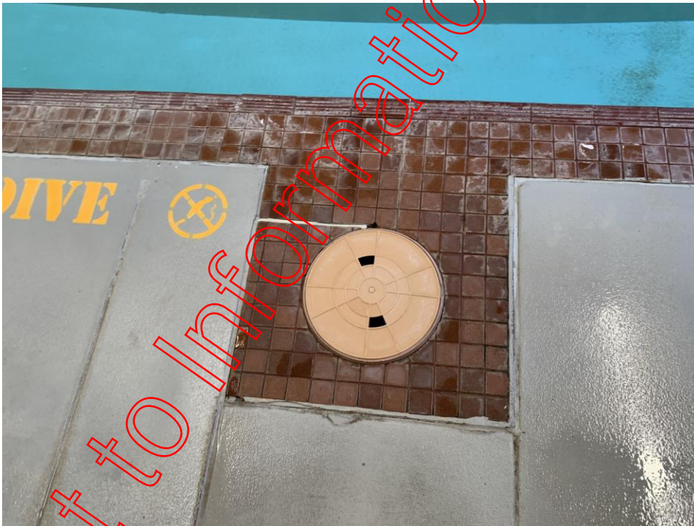
Figure 21: Skimmer in pool
