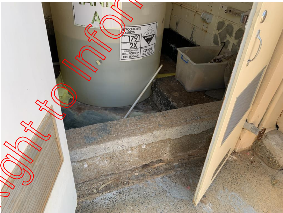
Figure 88: Poor condition bund wall
