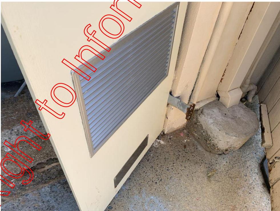
Figure 82: Failed door hinge, poor building condition
