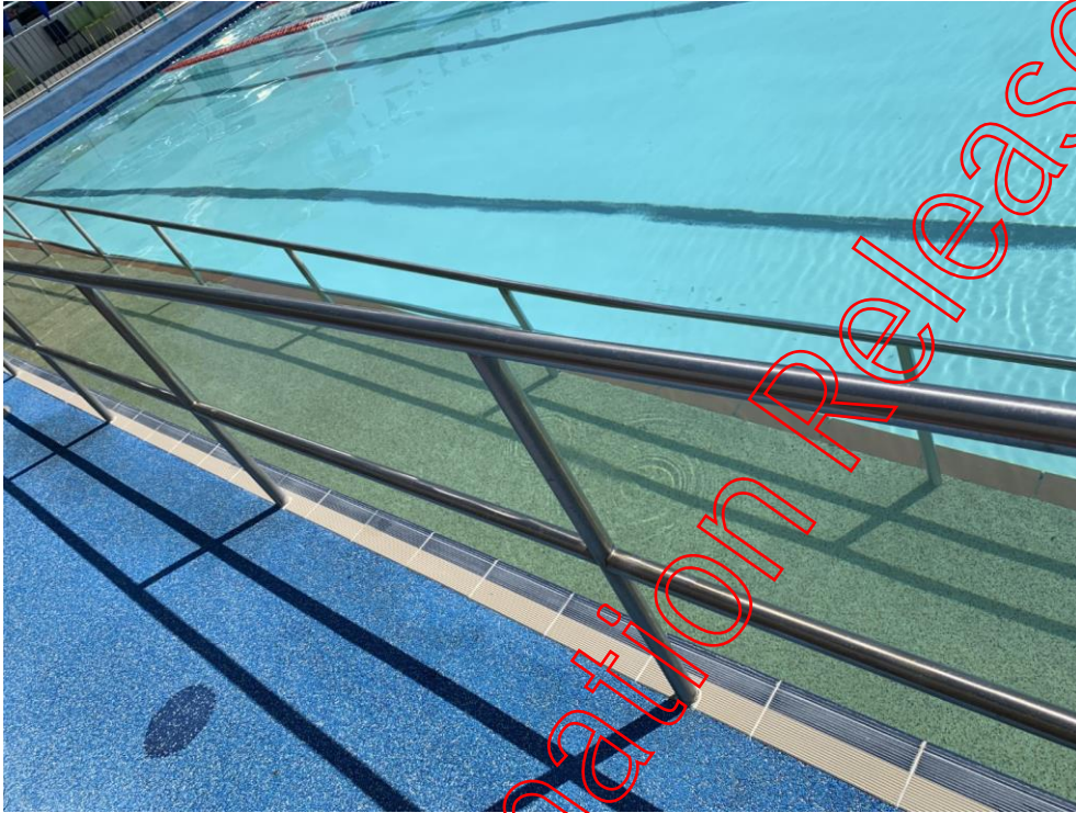
Figure 18: Lack of mid-landing in ramp
