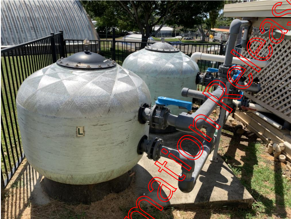
Figure 100: Pool filters with unsafe access, UV degradation to filters
