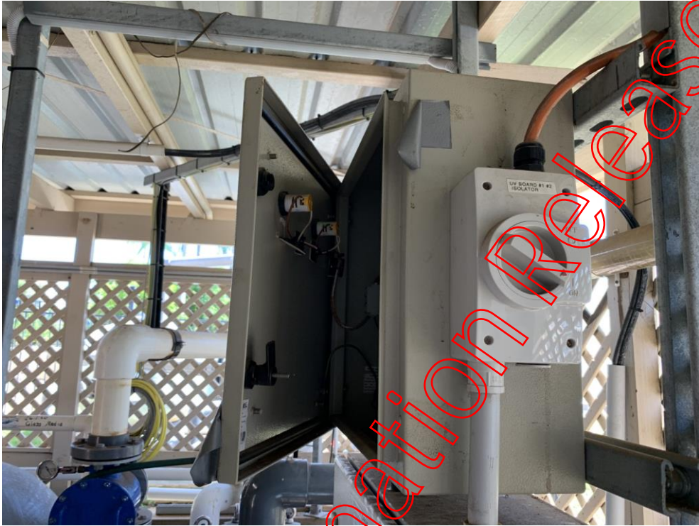
Figure 87: Open UV control panel with broken latches
