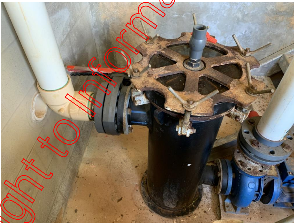
Figure 128: Filtration pump and strainer, poor condition, poor access, disused pipe
