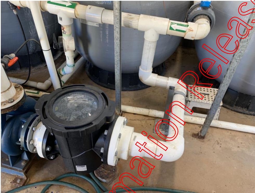
Figure 94: Restriction in filtration pump inlet
