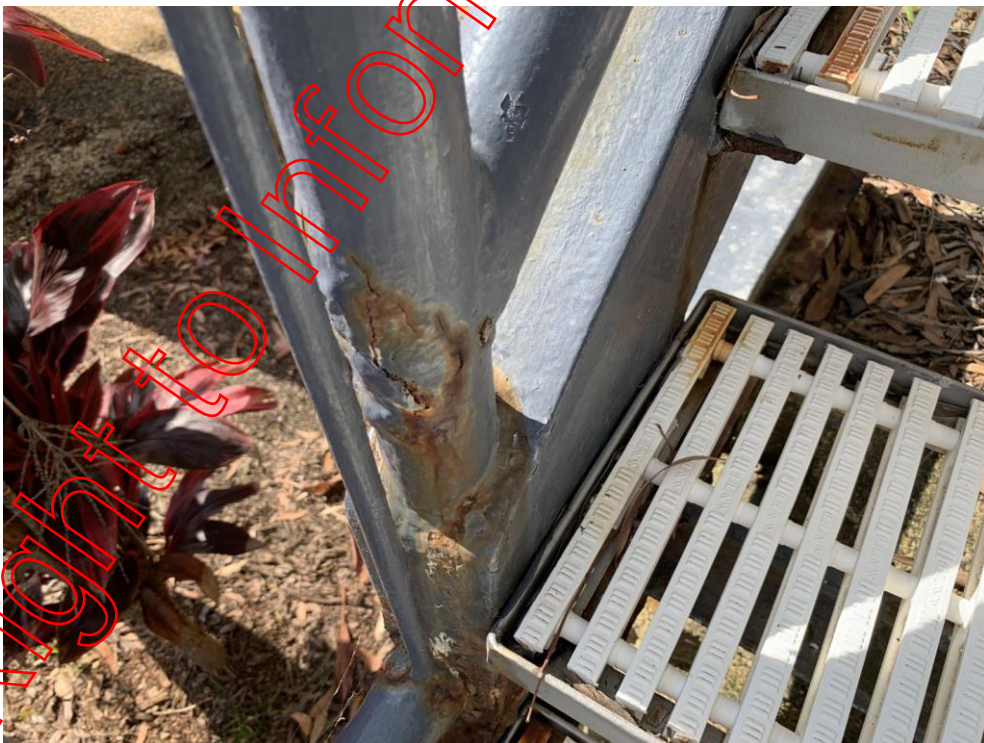
Figure 45: Rust in slide access way
