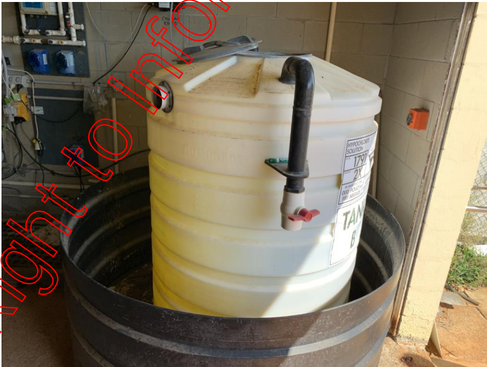
Figure 110: Chlorine tank with no fill point, overflow or level markings
