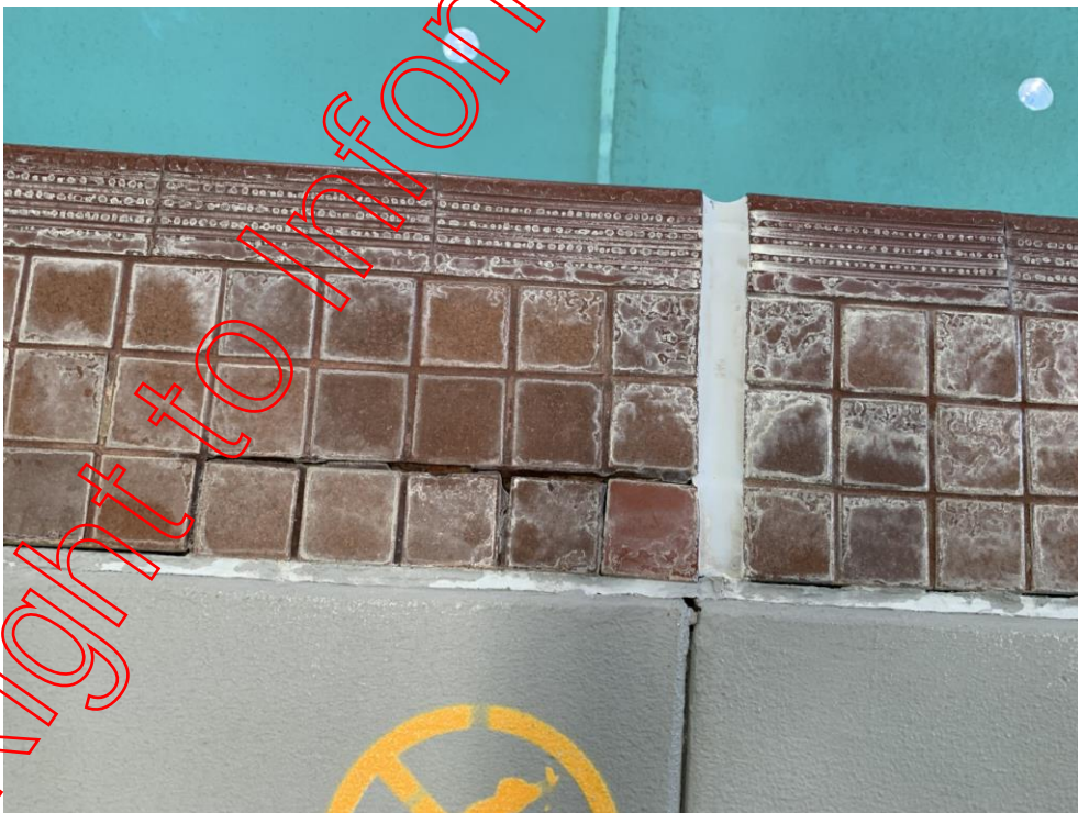
Figure 27: Degraded / damaged finishes
