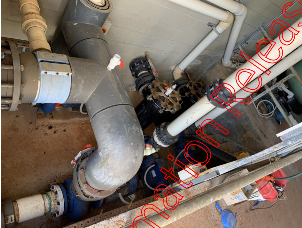
Figure 109: Submerged pump well, poor access
