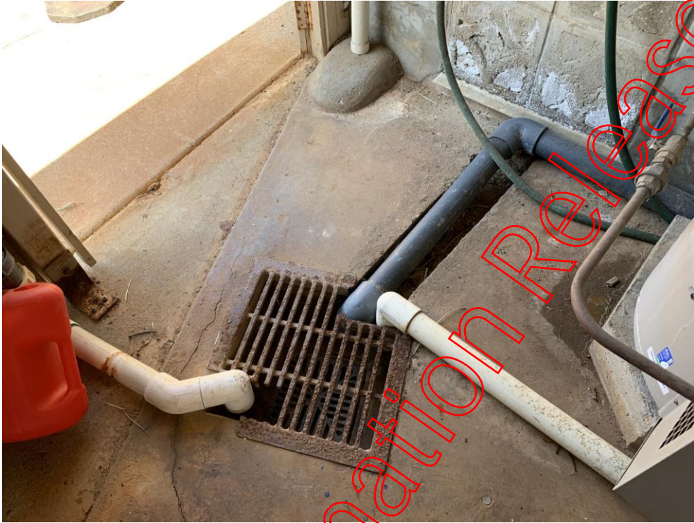
Figure 96: Backwash to floor drain, trip hazards
