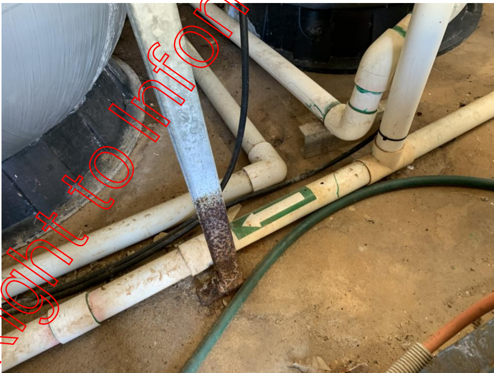
Figure 80: Rusted pipe supports, unsupported pipework
