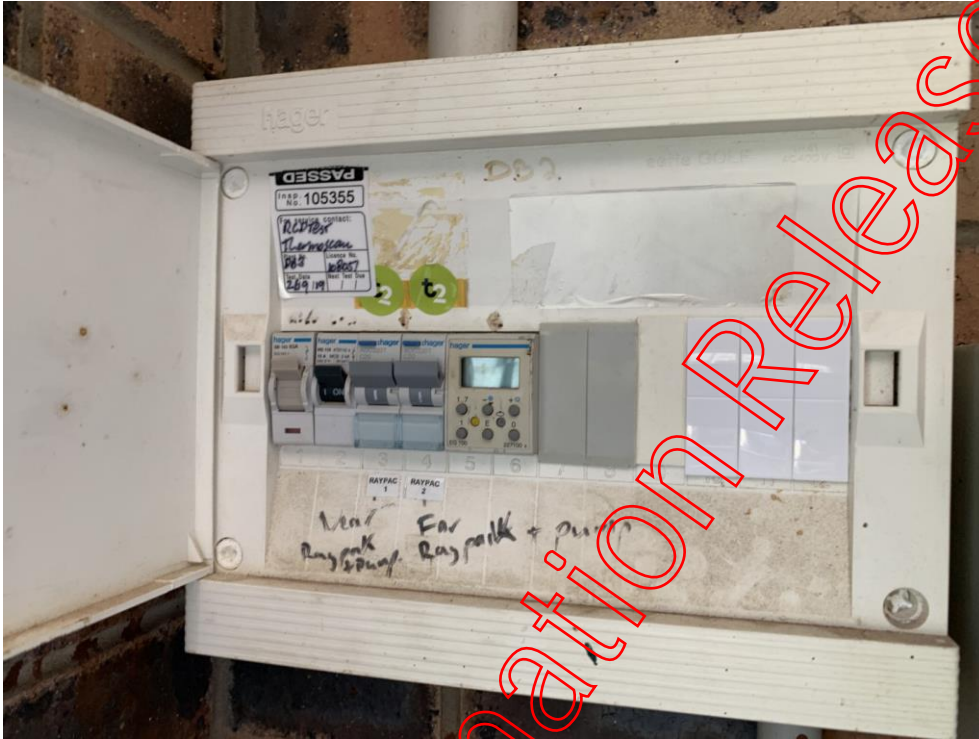
Figure 65: Poorly labelled control panel
