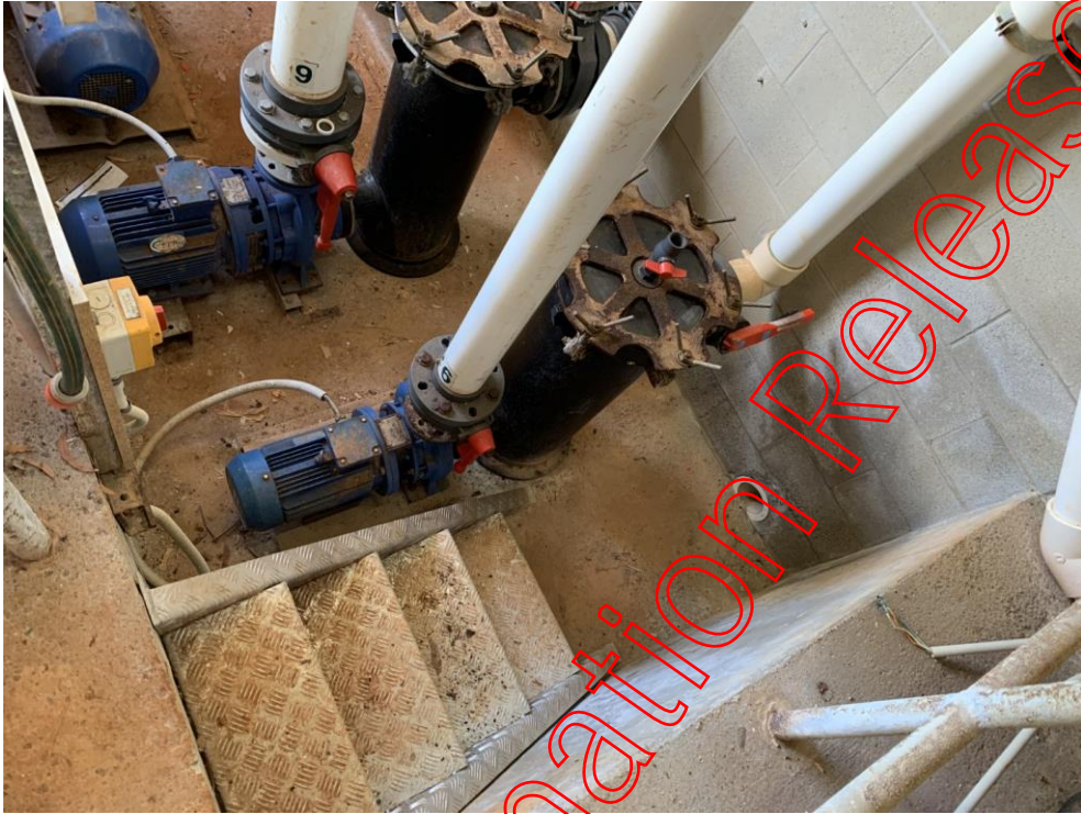
Figure 113: Stairway into pump well with no access at bottom
