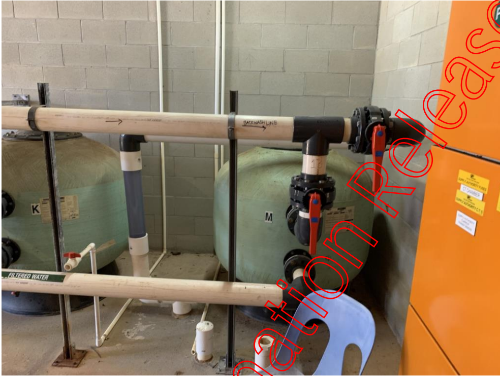
Figure 131: Spa filter incorporated into main manifold
