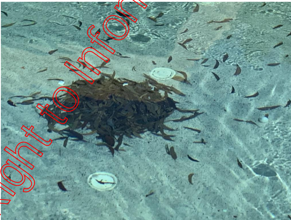
Figure 56: Debris accumulation in pool
