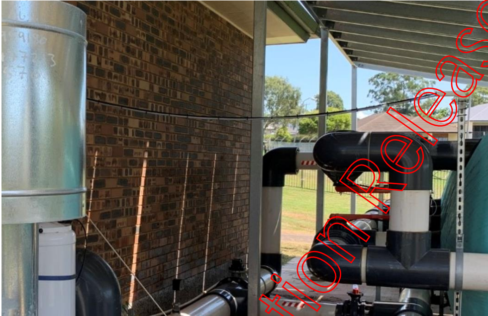
Figure 73: Unprotected dosing line suspended between wall and bracket
