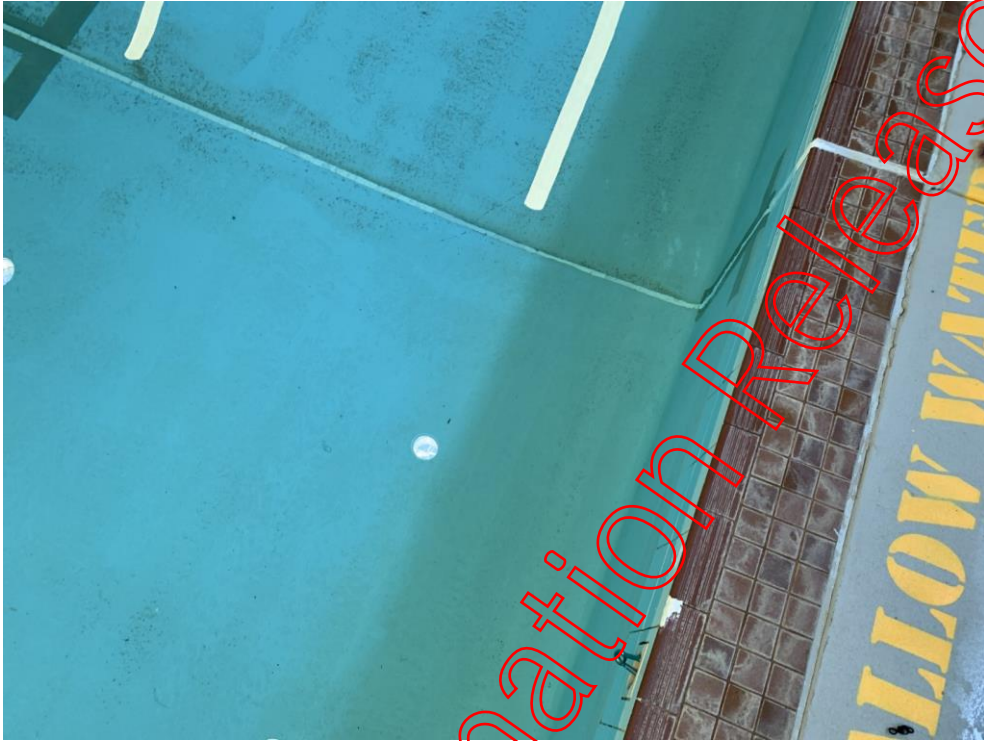
Figure 22: Failing finish on floor of pool
