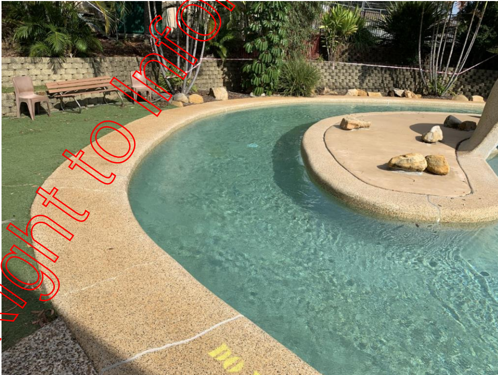
Figure 48: Cracks in coping
