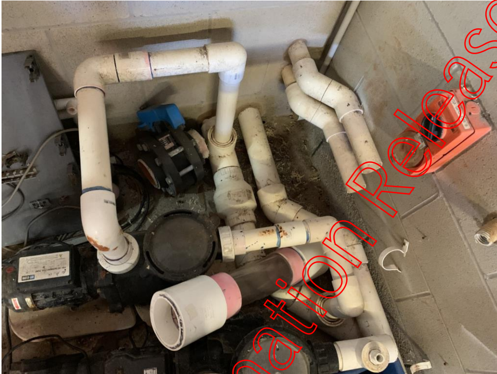
Figure 115: Obsolete equipment, poorly labelled pipework, disconnected heater pipework
