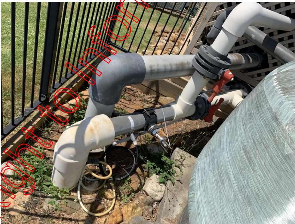
Figure 105: Chlorine injection point
