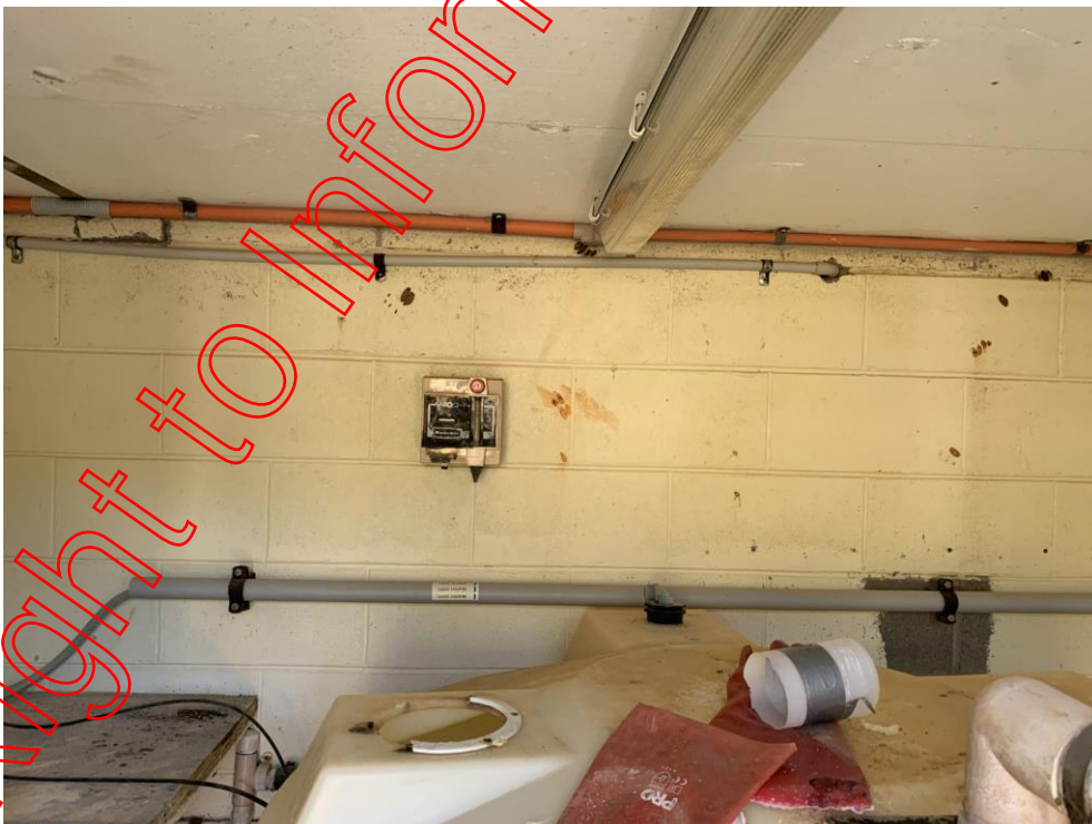
Figure 92: Disused equipment, open inlet to tank
