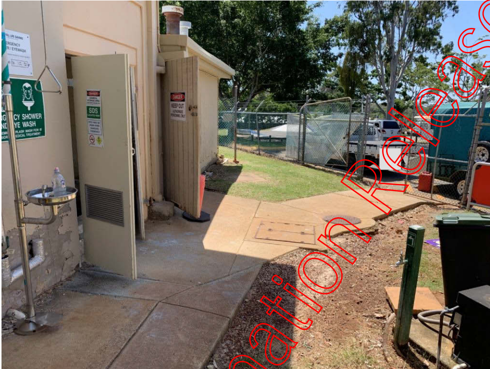
Figure 85: Unsafe working surface between plant and truck unloading area
