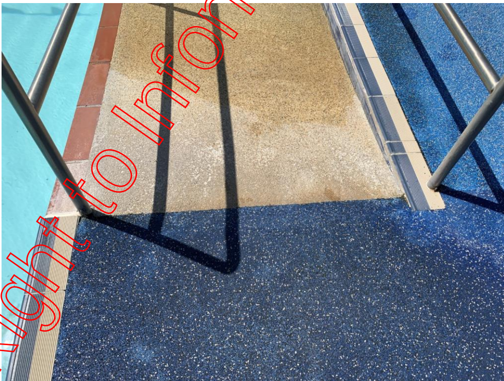
Figure 19: Initial transition into ramp identified as slippery
