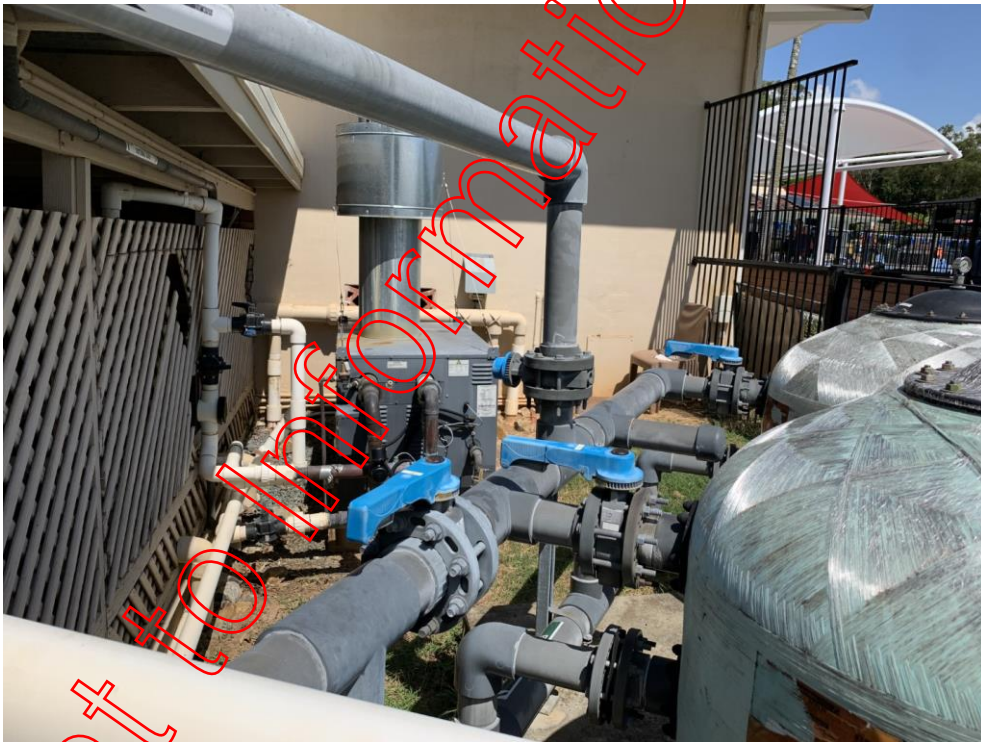
Figure 76: Poor condition external equipment, unsafe access to manifold
