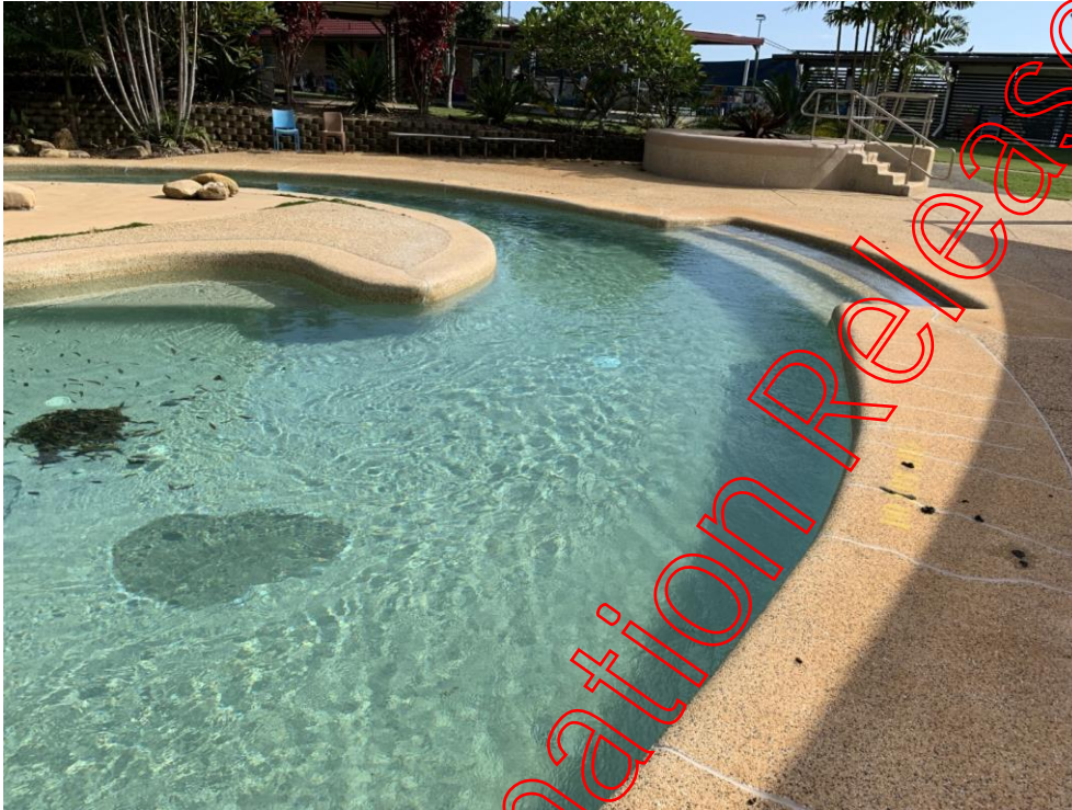
Figure 49: Cracks in coping, missing floor finish
