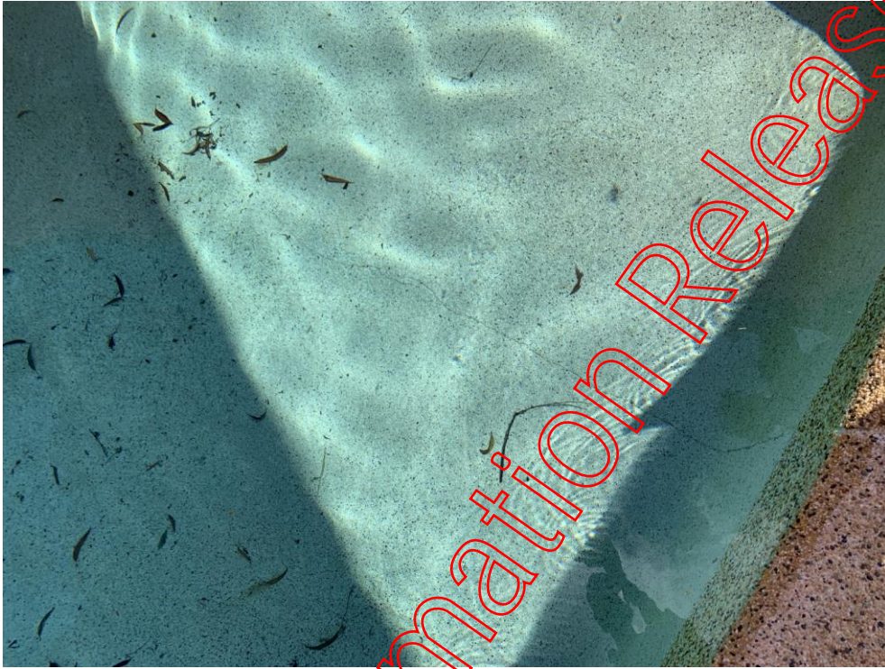
Figure 29: Crack across pool floor on eastern side
