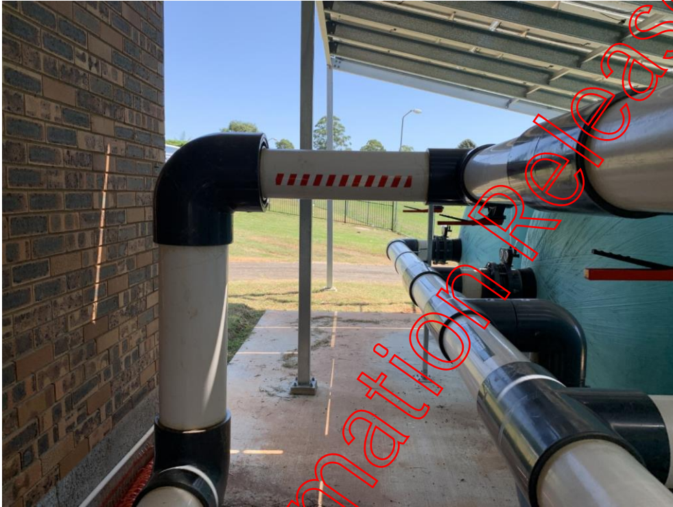
Figure 67: Premature step down of pipe size, head strike
