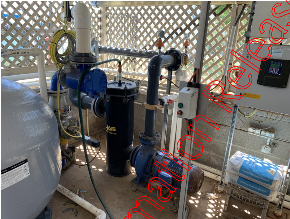
Figure 99: LTS Pool Pump and UV Unit
