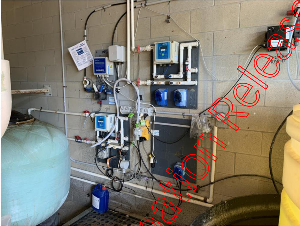
Figure 111: Chemical control and dosing area with disused equipment
