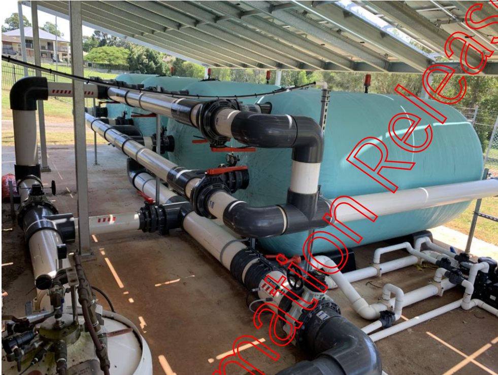
Figure 66: 50m Pool Filters
