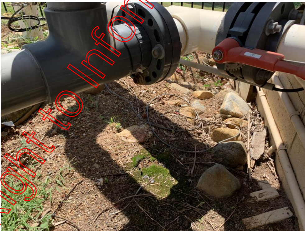
Figure 103: Leak in pipework
