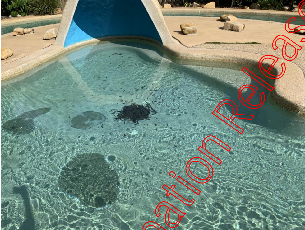
Figure 55: Missing floor finish
