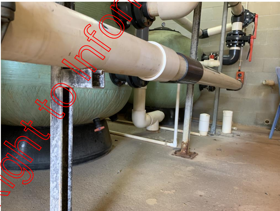
Figure 118: Inadequate pipe supports in filter manifold
