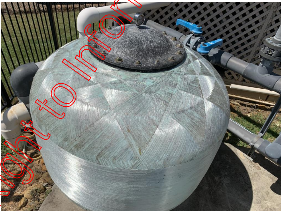
Figure 107: UV degraded filter
