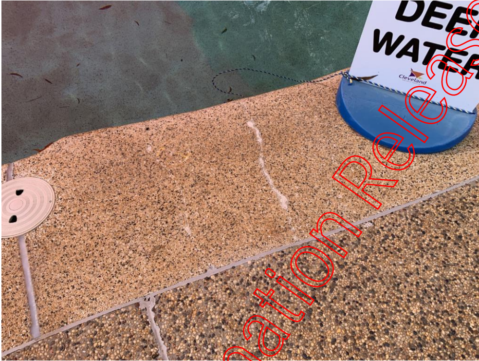
Figure 31: Cracks in coping
