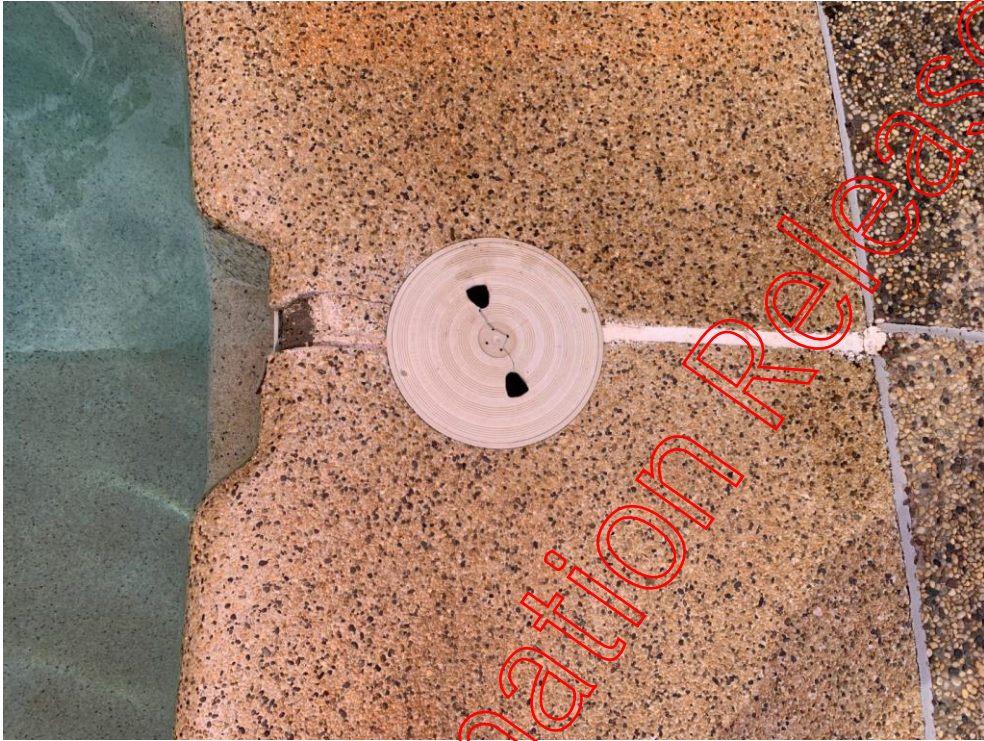
Figure 33: Broken skimmer lid
