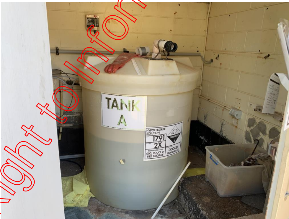
Figure 90: Tank with no level markings or solid plumbing connections
